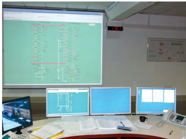
Control room at the Kyiv 750kV substation
