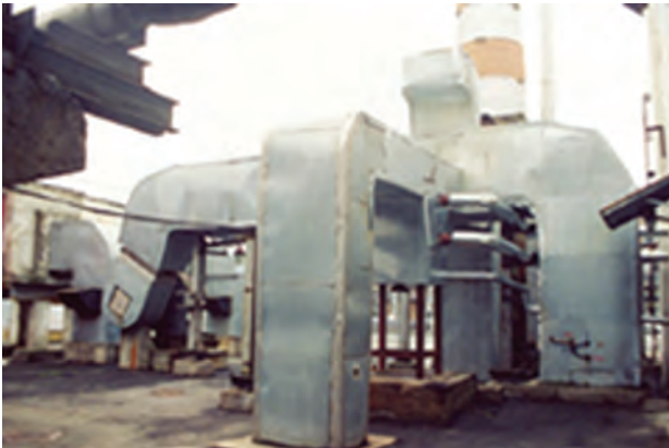
Heat recovery plant with TPK-1.1-230 regenerator installed behind DE-16-14GM boiler at the boiler house of Farmak corporation, Kyiv
