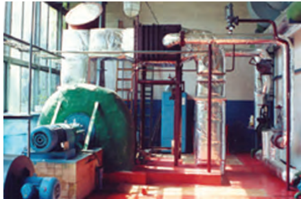
Heat recovery plant with convection bank PK-1-102 sh installed behind TVG-4r boiler at the boiler house at 2a Osipovska St., Kyiv
