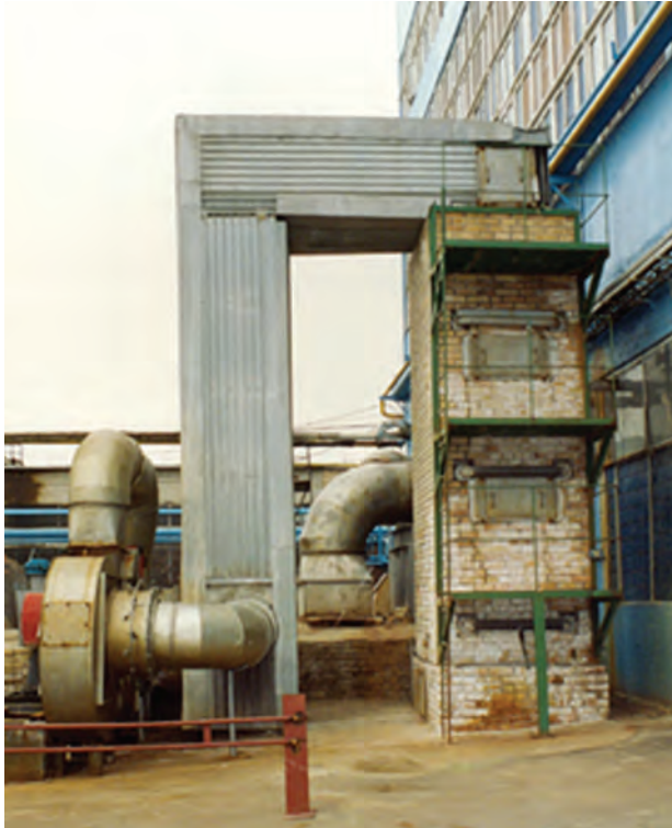
Heat recovery plant with TVM regenerator installed behind the furnace No. 3 of Hostomel Glassworks in Kyiv Oblast
